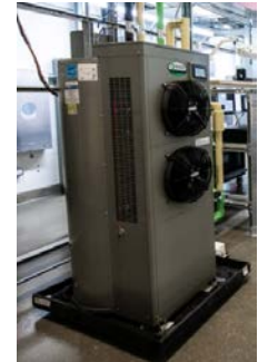
Photo by Dennis Schroeder NREL 62043
